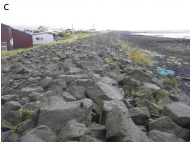
Figure 4. Former strategies to cope with periodic flooding in Eyrarbakki and Stokkseyri, in southern Iceland, involved a sacrificial basement with living quarters reached via steps (A, B). Subsequent construction of dykes (C) to control flood risk has led to permanent occupation of these basements. The community has thus moved from a situation where they lived with floods to one where they actively resist them. Permanent occupation of the lower levels of buildings means that when flooding happens it will be much more damaging than before.
